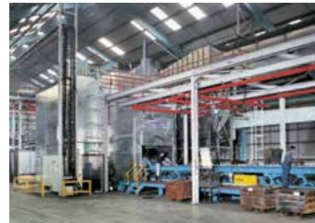
CT-6 blast cleaning machine with noise abatement cabin and sorting belt
