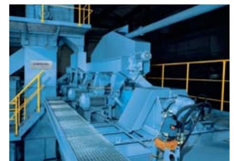
Cabin top of a DT 14-1050 equipped with 10 blast wheels
